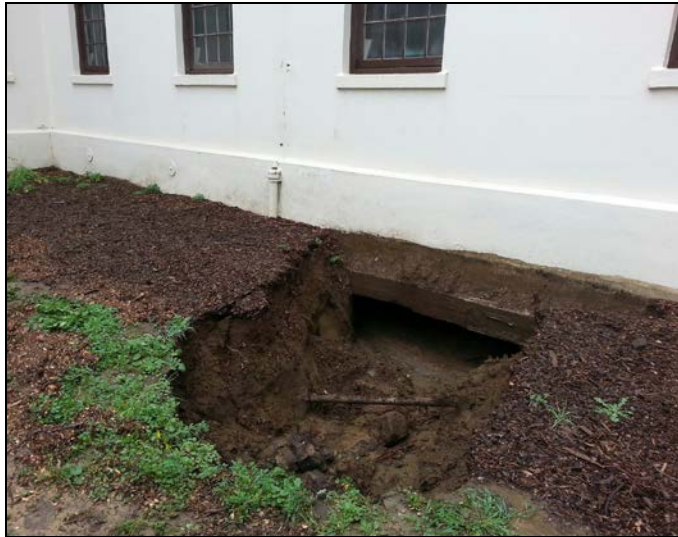
Heavy rains and poor drainage systems led to erosion and destabilization of building 650's foundation pictured here on February 9, 2014.
