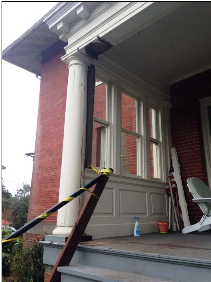
The porch at Infantry Terrace building 333 with one intact column in place and an identical adjacent column removed because of extensive dry rot. Trust carpenters worked with an outside shop to reconstruct a replacement column that matched materials and assembly of the original. (2014)
