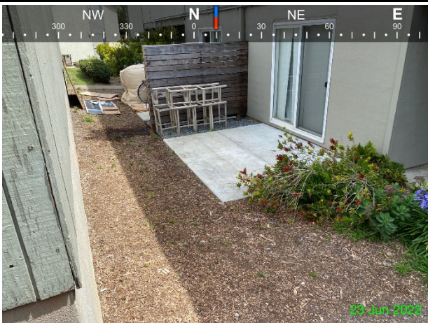
Photo 11: 6/23/2022 – View of intact concrete patio and soil cap to the west of Building 1278.
