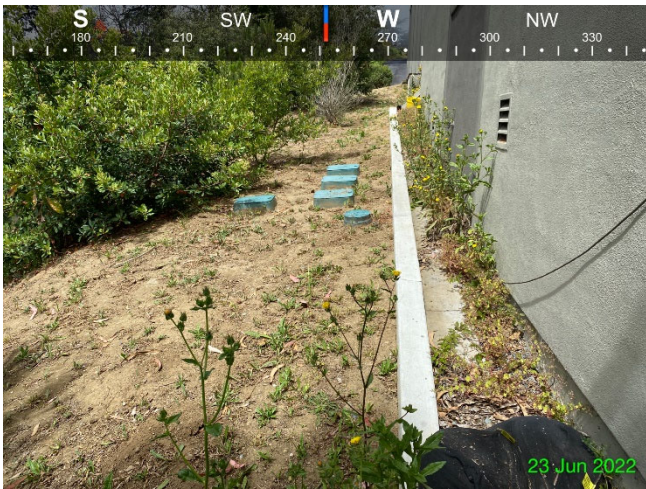
Photo 9: 6/23/2022 – View of intact hardscape and vegetated slope to the south of Building 1259.
