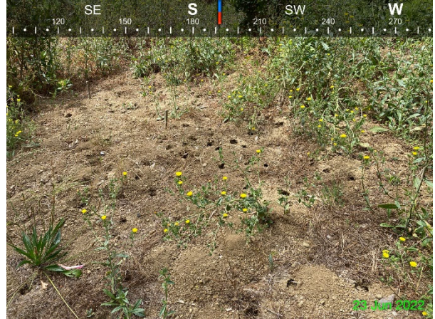
Photo 4: 6/23/2022 – Area of bare exposed earth where burrowing activity is present in the area between Buildings 1278 and 1279.
