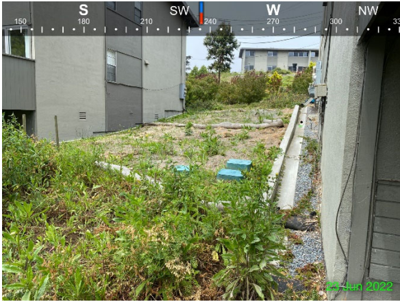
Photo 7: 6/23/2022 – View of erosion protection between Buildings 1278 and 1259. Intact hardscape and drainage shown from the southeast corner of building 1278.
