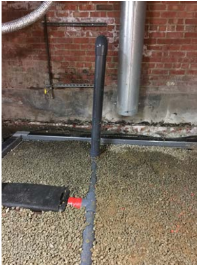
Photo 9: Fresh Air Intake
