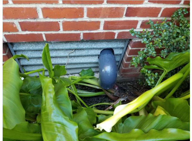
Photo 32: Fresh Air Intake
