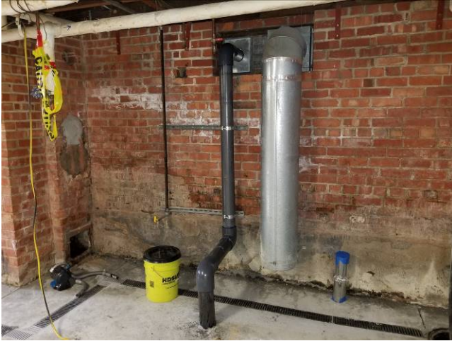
Photo 31: Fresh Air Intake
