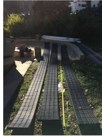
Photo 2: VMS subsurface piping
