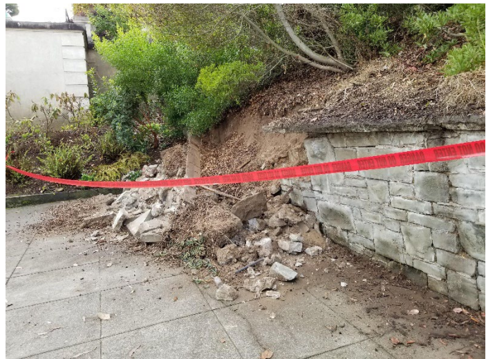
FIGURE 5: LYON-VALLEJO BOUNDARY WALL COLLAPSE, NOVEMBER 2020
