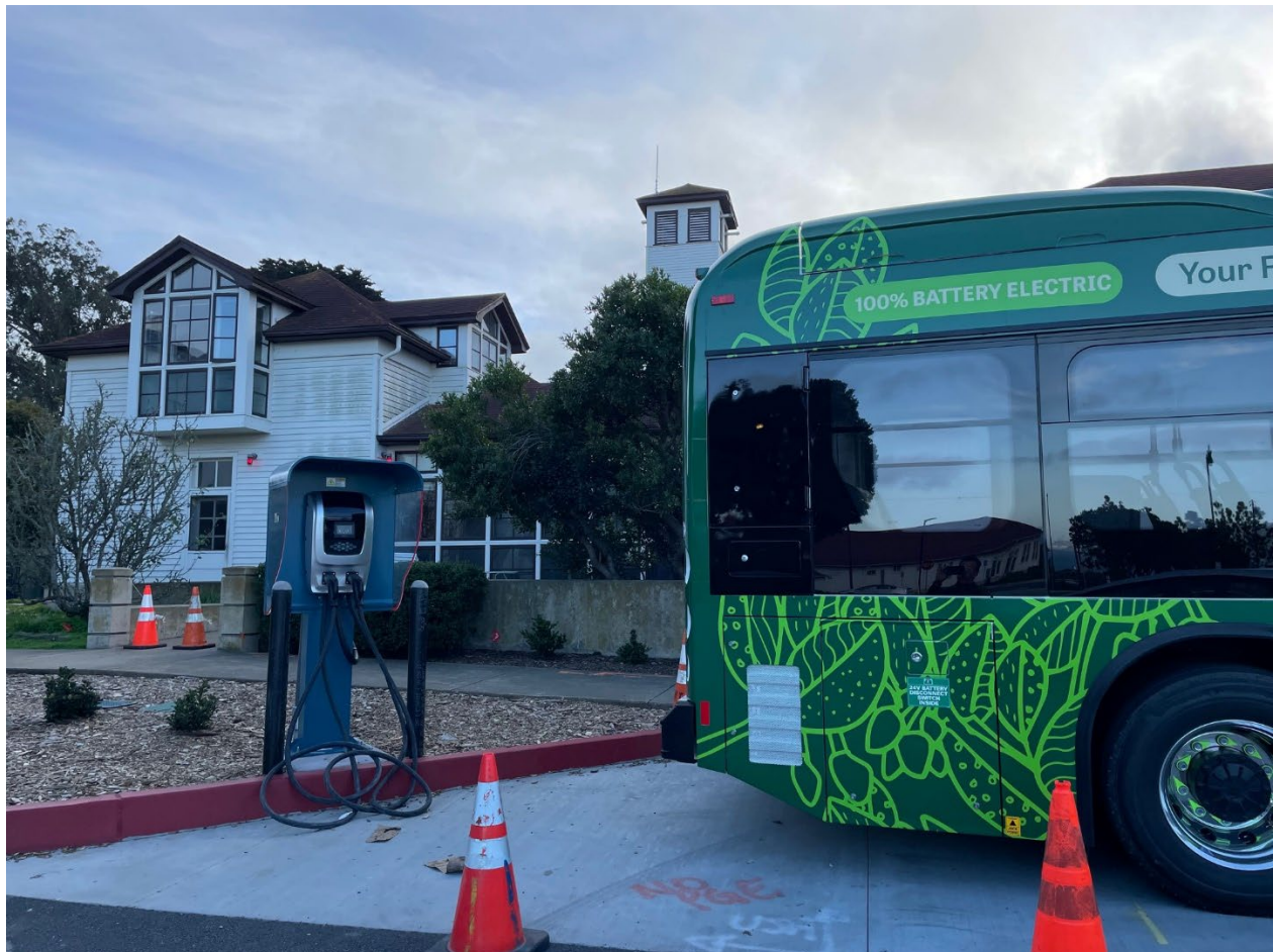
FIGURE 8: ELECTRIC BUS CHARGING STATION
