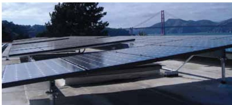
PHOTOVOLTAIC PANELS ON BUILDING 211
