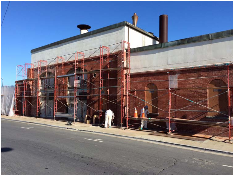
Paint stripping underway at building 1040 as part of the larger preservation maintenance program in the Thornburgh District.
