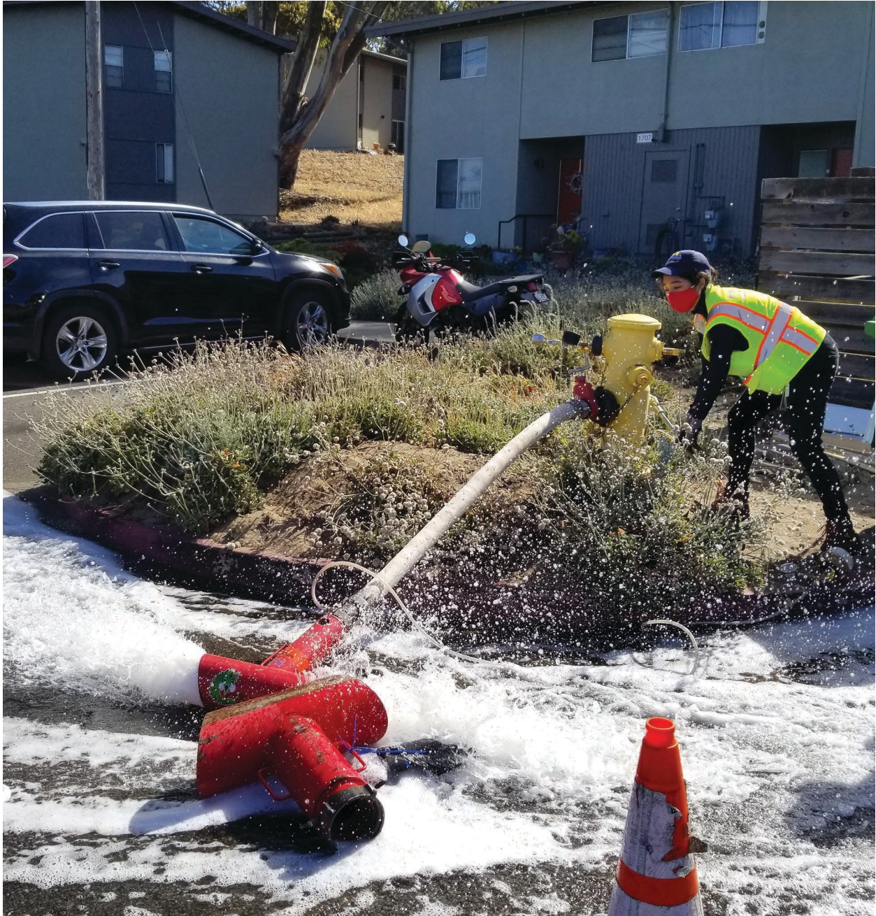
Flushing our system park-wide in order to gather flow, and pressure data
