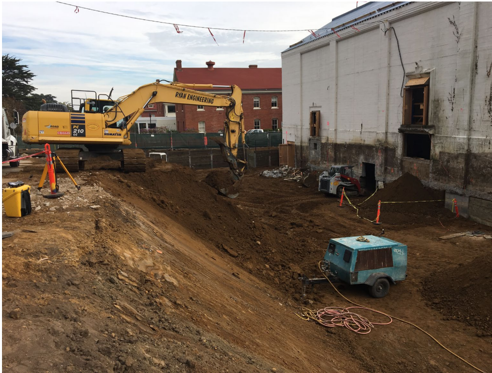
Figure 2 Excavation for the below grade portion of the project (Presidio Trust, January 2018)
